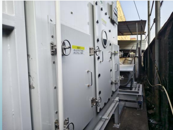
Image: A newly built “Dry Filtration facility / Zeolite Rotor Concentrator” by a company in Hunan
