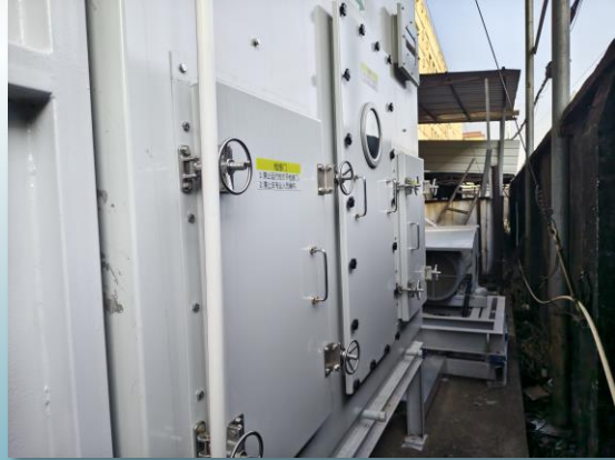
Image: A newly built “Dry Filtration facility / Zeolite Rotor Concentrator” by a company in Hunan
