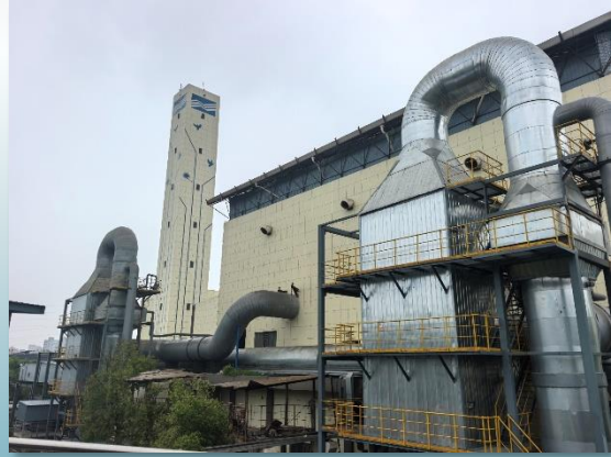
Image: A newly installed flue gas SCR denitrification facility by an enterprise in Zhejiang
